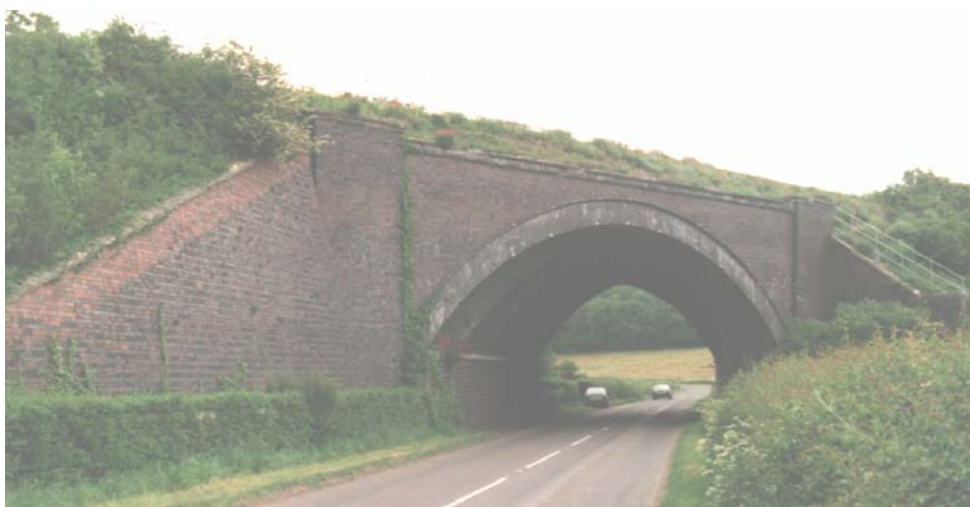
A bridge near Somerton, the GW line avoiding Bristol Note this bridge is unusual as the embankment continues across it.
